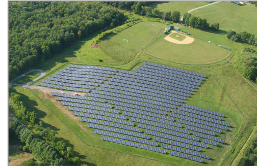
Sullivan Solar Garden 2 MW | Loch Sheldrake, NY PPA: SUNY-Sullivan College
